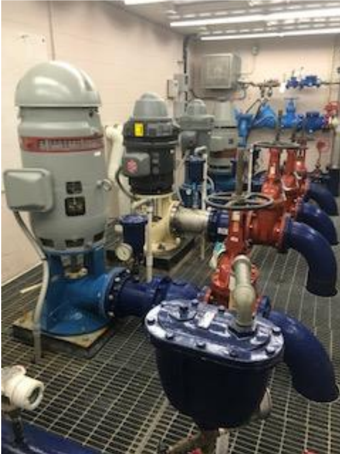
High Lift Pump House
