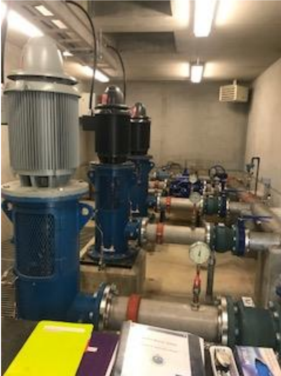
Bayview Booster/PRV Station
