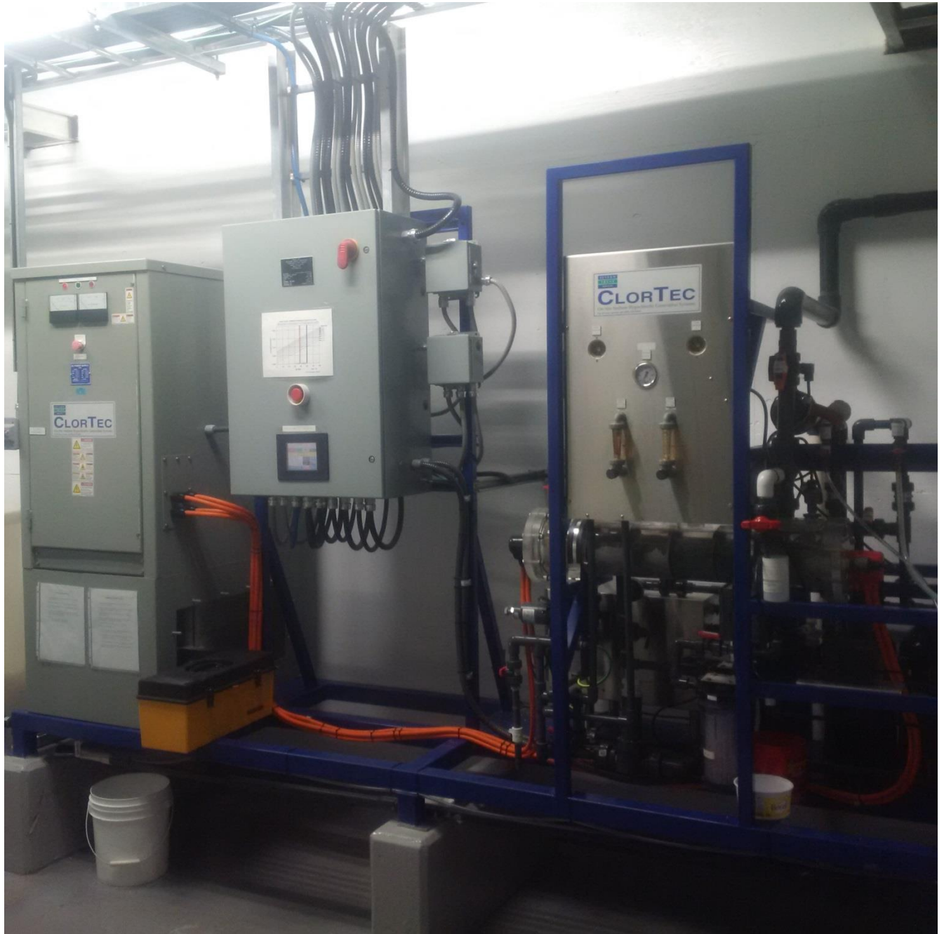
Sodium Hypochlorite Generator
