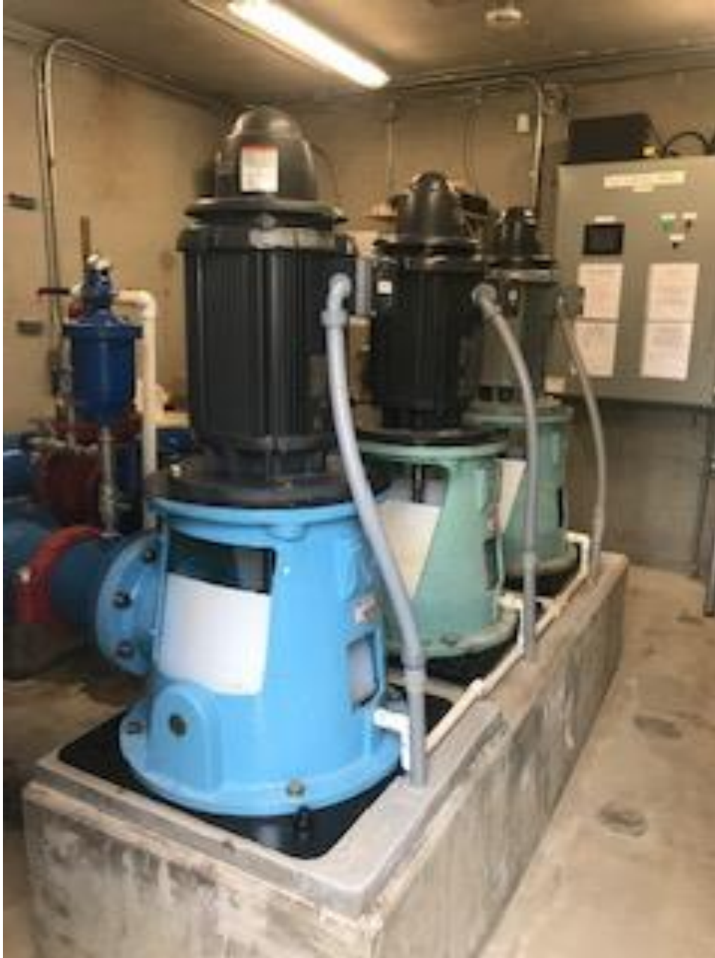
Low Lift Pump House
