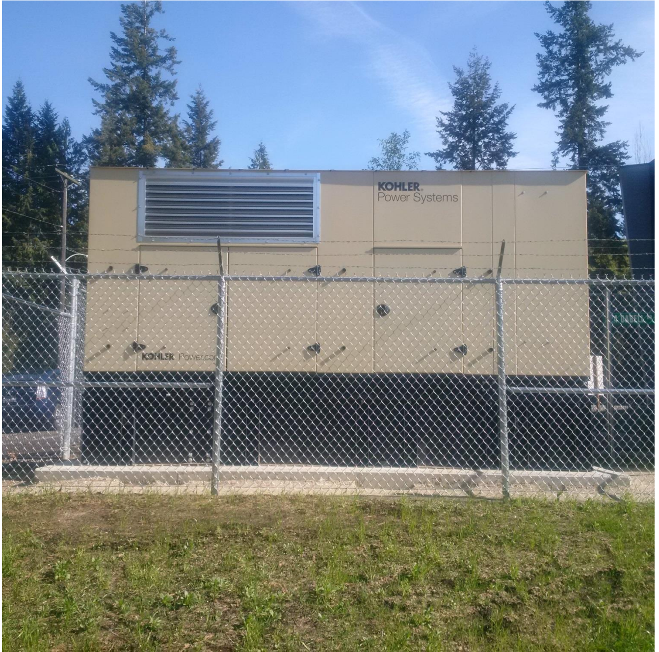
WTP / High Lift Pump House Generator
