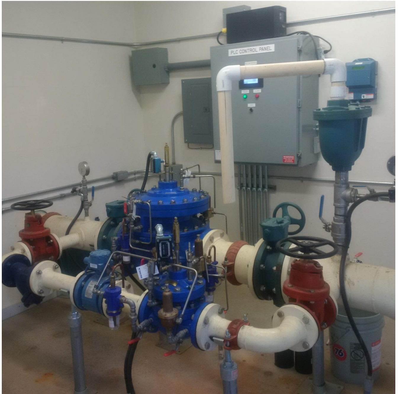
Two Mile PRV Station
