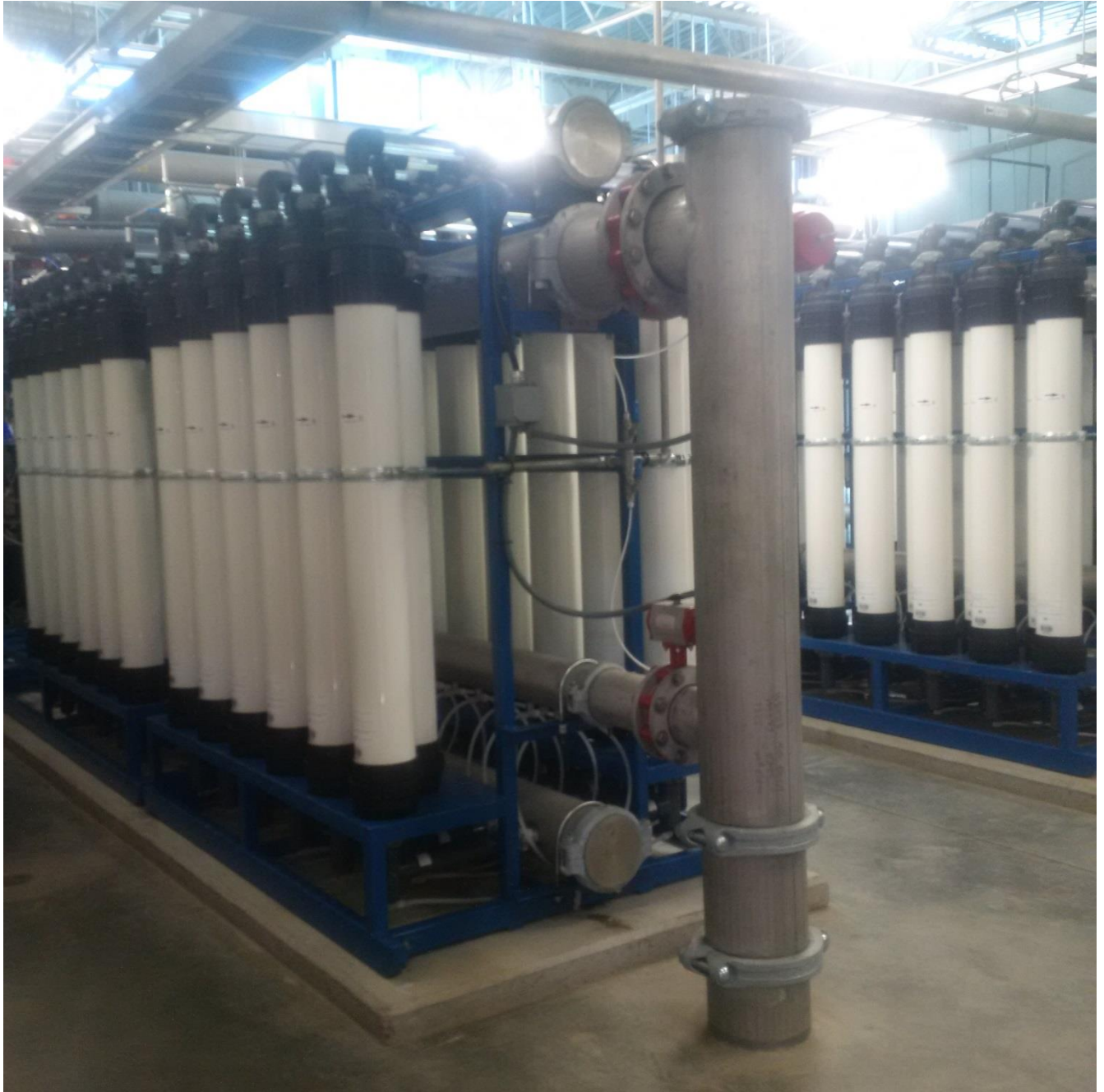
Water Treatment Plant
