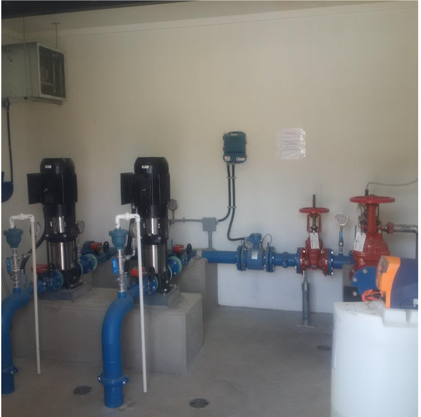
CPR Hill Booster Station
